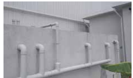
Waste Water Management System at the Muthurajawela Warehouse
